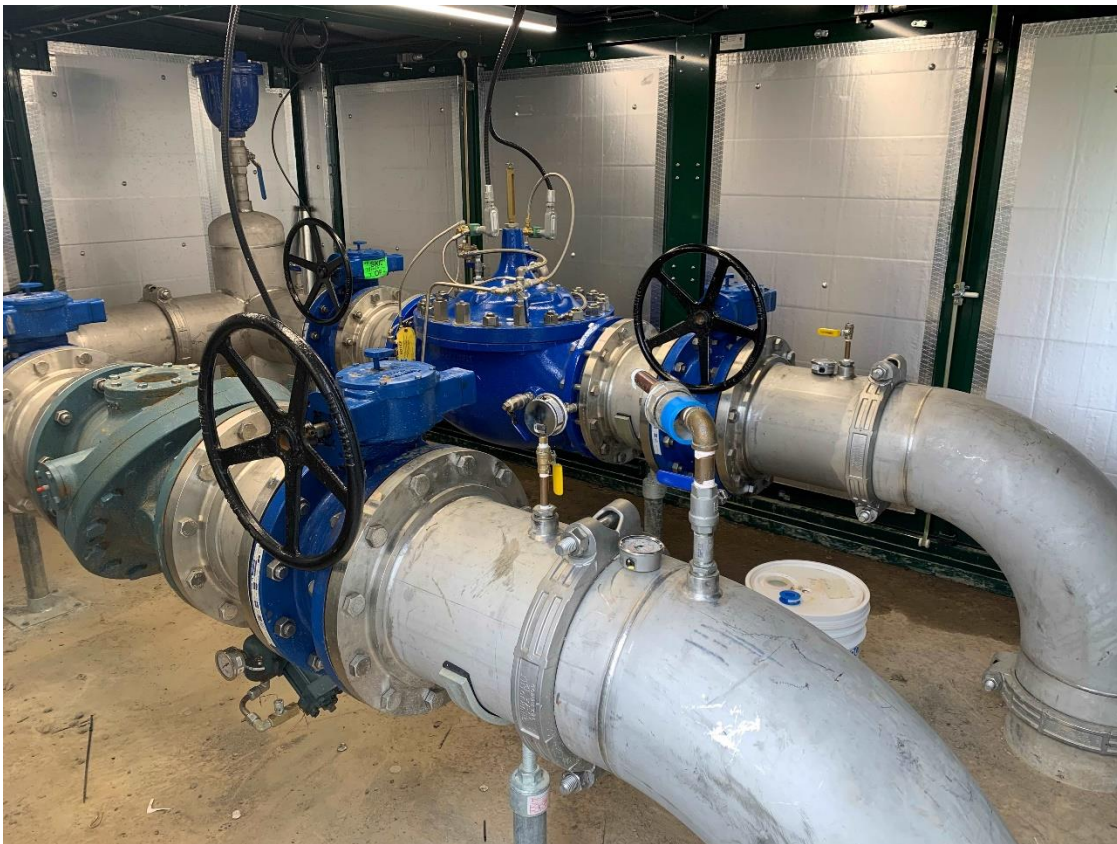
IMAGE | WATER INFRASTRUCTURE AT THE RESERVOIR SITE.
