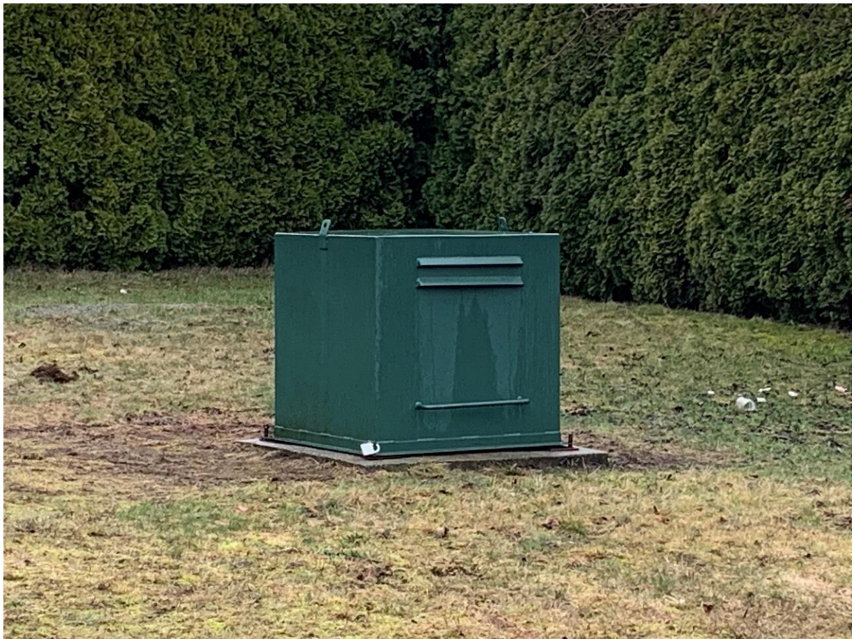
IMAGE | RW 1-87/14 WELLHEAD COVER.
